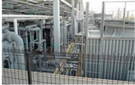
System harvests heat from reclaimed wastewater
